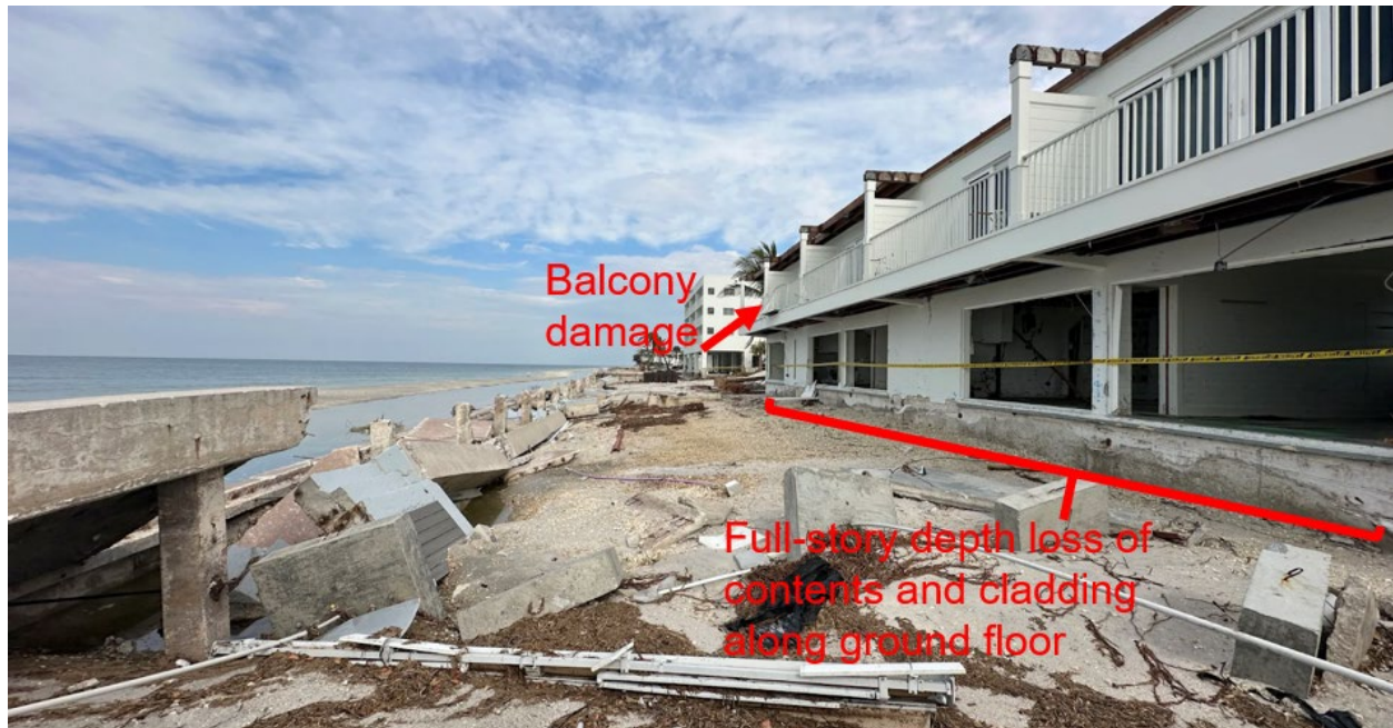
Figure 7.1. Seawall failure associated with storm surge in Manasota Key; depth of storm surge evident from loss of ground floor unit cladding and contents suggesting storm surge to full height of ground floor (Source: Mike Lang/Sarasota Herald Tribune ).
