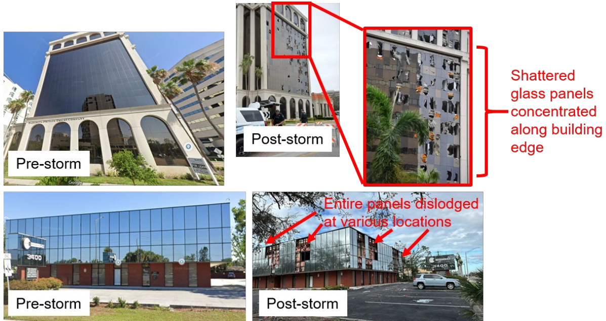
Figure 4.5. Shattered glass panels at Sarasota Private Trust Company (top) and dislodged window panes at Sarasota Retina Institute (Sources: Top left and middle Mike Lang , top right, bottom left, and bottom right: Derek Gilliam ).
