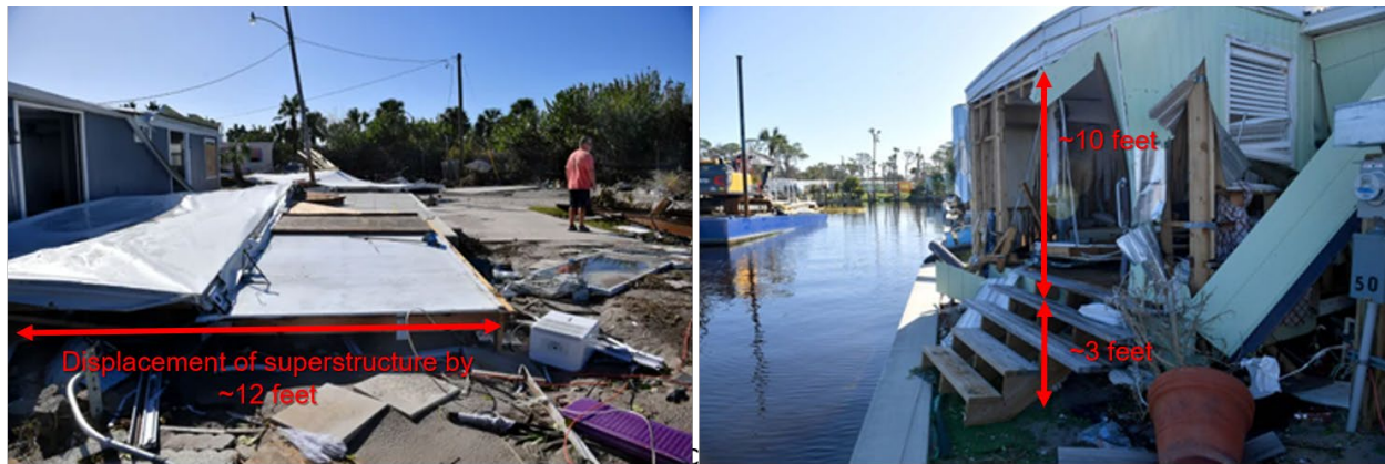
Figure 4.8. Destruction of mobile homes in Shady Haven Mobile Home Park in Englewood, FL, caused by storm surge: (left) mobile home displaced 12 feet from foundation; (right) mobile home also displaced from its foundation with severe wall damage from storm surge (Source: Mike Lang/Sarasota Herald-Tribune ).
