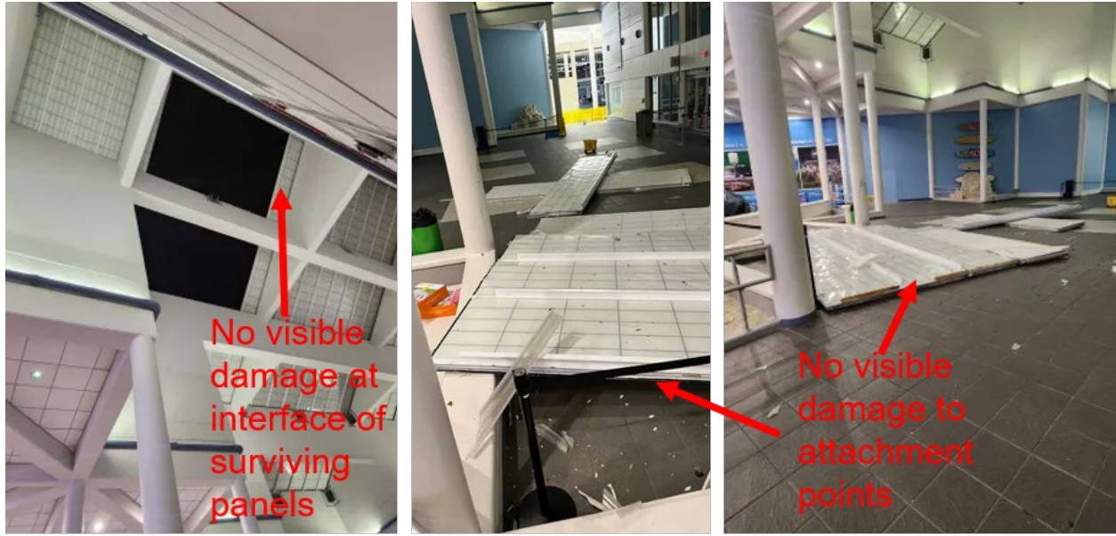
Figure 4.6. Skylight failures at Melbourne Orlando International Airport where entire skylight panels were apparently unseated under wind gusts. No visible damage to the panels or their attachments is apparent (Source: Jennifer Sangalang/USA TODAY NETWORK ).
