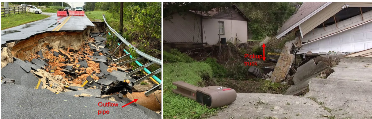
Figure 6.1. Example of geotechnical failures in Hurricane Milton (left) collapse of Wolf Branch Road at Niles Road in Mt. Dora adjacent to body of water receiving outflow; (right) sinkhole between two residences in Polk County, swallowing a pick up truck and leading to partial collapse of garage (Source left: Daily Commercial ; Source right: Bowen, 2024).
